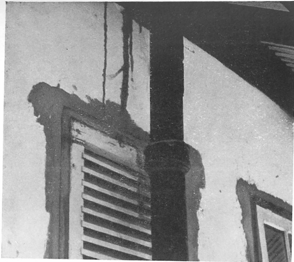
Covered runways of earth constructed by termites on a wall leading from an infested wall plate down to a newly-fitted louvre-window. They had reached the roof through wall cracks in another part of the building.
